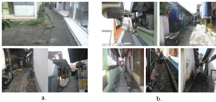
Figure 4. a. With drainage and not yet equipped with drainage; b. Roads with broken pavement (paving, concrete) and ground (Source: photograph by author,2017)
